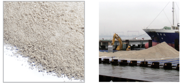
写真8 土工用水砕スラグと岸壁での施工例 Photo 8 Water granulated slag for civil engineering works and example of construction for quay
